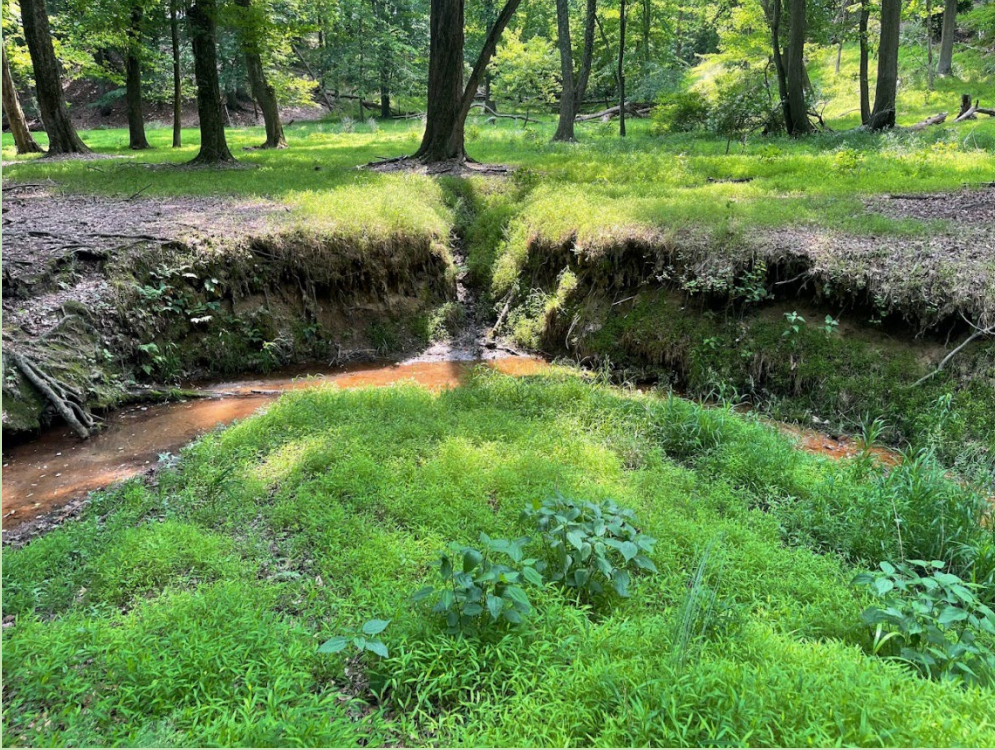
Unstable outer meander, showing headcut forming in floodplain below lateral ravine entering floodplain, effectively draining seep wetland above.
