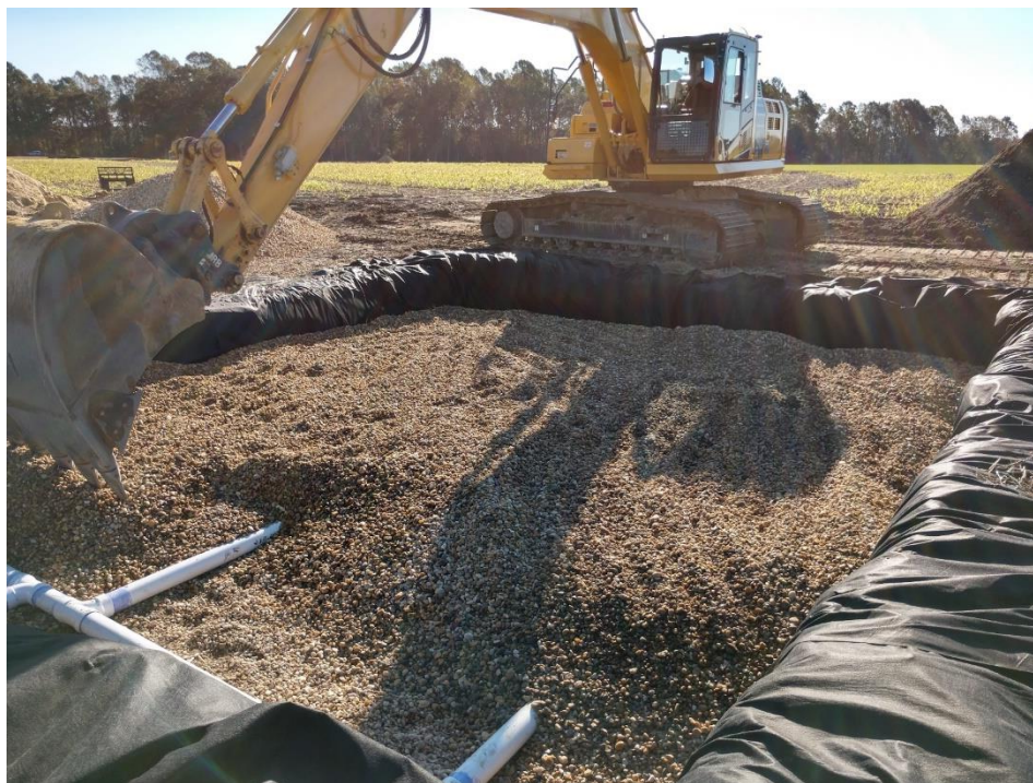
Figure 4: Blind inlet example showing the filter (gravel) being placed over the subsurface perforated drainage pipes.
