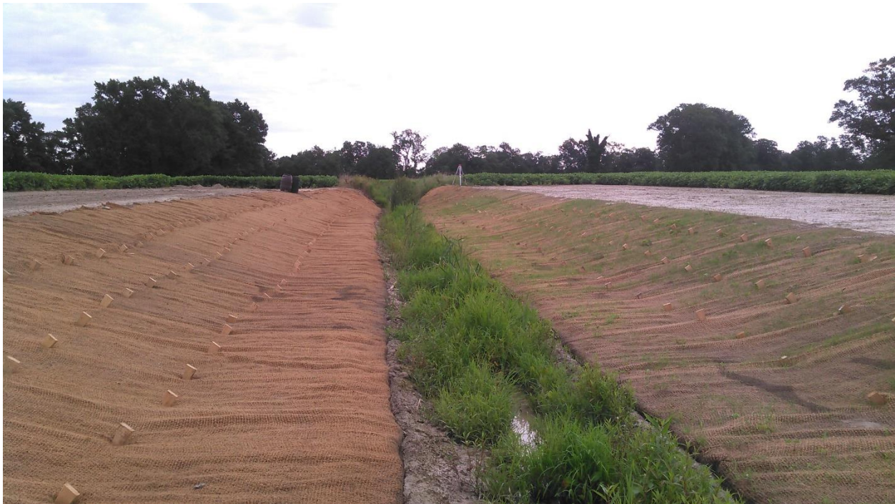
Figure 13: Two-Stage Ditch example showing the extended benches within the ditch. This two-stage ditch is located in Talbot County, MD.
