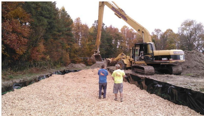
Figure 6: Denitrification Bioreactor example showing the subsurface woodchip-filled pit.
