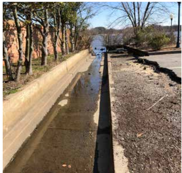
A town founded in 1706 means much of the stormwater infrastructure is outdated or historical. Top: an old stormwater pipe drains directly to the river. Bottom: the infamous drainage ditch at the end of High Street empties into the Chester. Pipes and ditches like these all over Chestertown dump stormwater, trash, fertilizer, chemicals, and more into the Chester River without any treatment.
